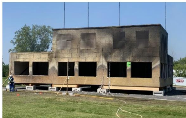
State of mass timber structure after fire research test.
